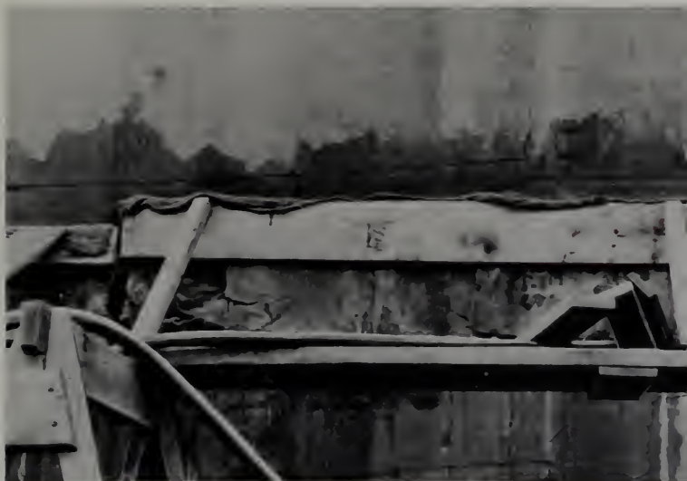
Figure 179.—Moist curing of surfaces of concrete repairs by supporting burlap mats against them. Wetting the burlap twice a day is usually sufficient to keep the surface continuously wet in this excellent method of treatment. (See also Figure 178.) (PX-D-33059.)
